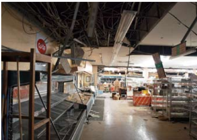
Co-op Mart Kunimi of Co-op Fukushima, with the ceiling down and the wires hanging visibly.
