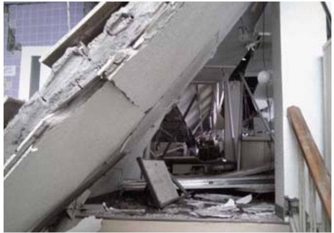
Inside the Miyagi Co-op Head Office Building "A," which was heavily damaged.
