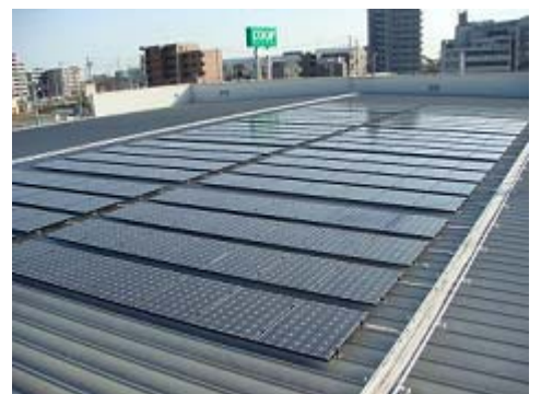
Solar panels installed on Tomizawa Store (Miyagi Co-op)
