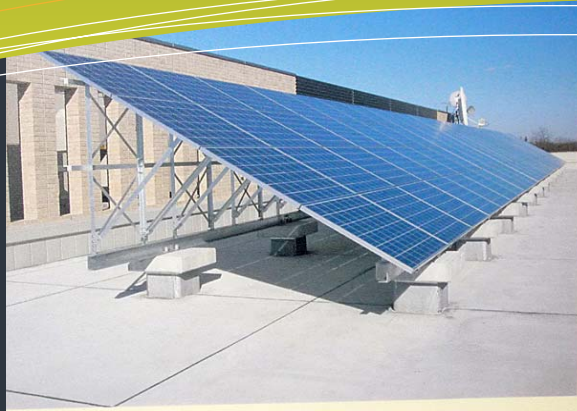
Rooftop / Photovoltaic system (converts solar radiations into direct current electricity)
