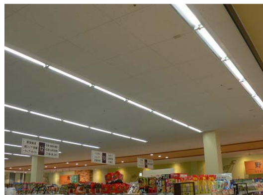
Using high efficiency light reflector to improve illumination intensity in the store.
